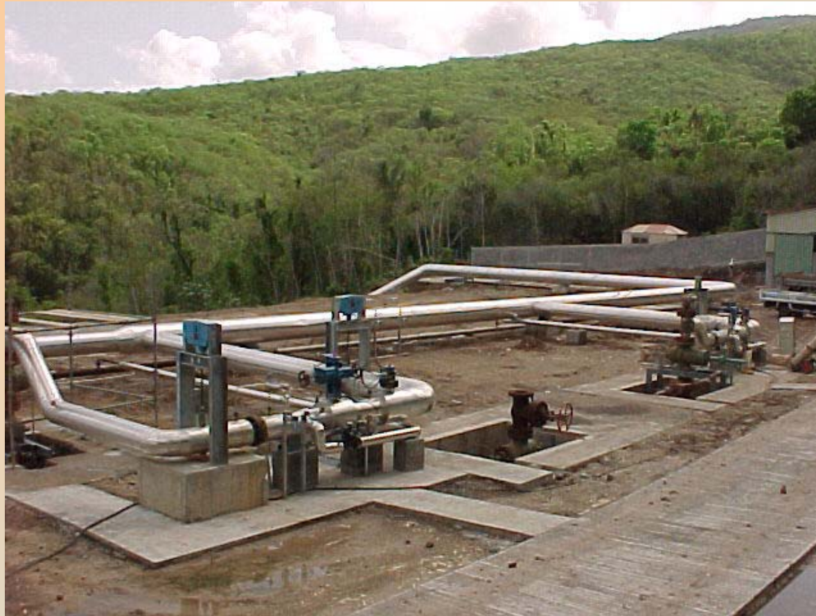
Partial view of the well pad with four well heads BO-4 to BO-7, at the end of the construction work and of the geothermal fluid transportation pipe to the power plant
